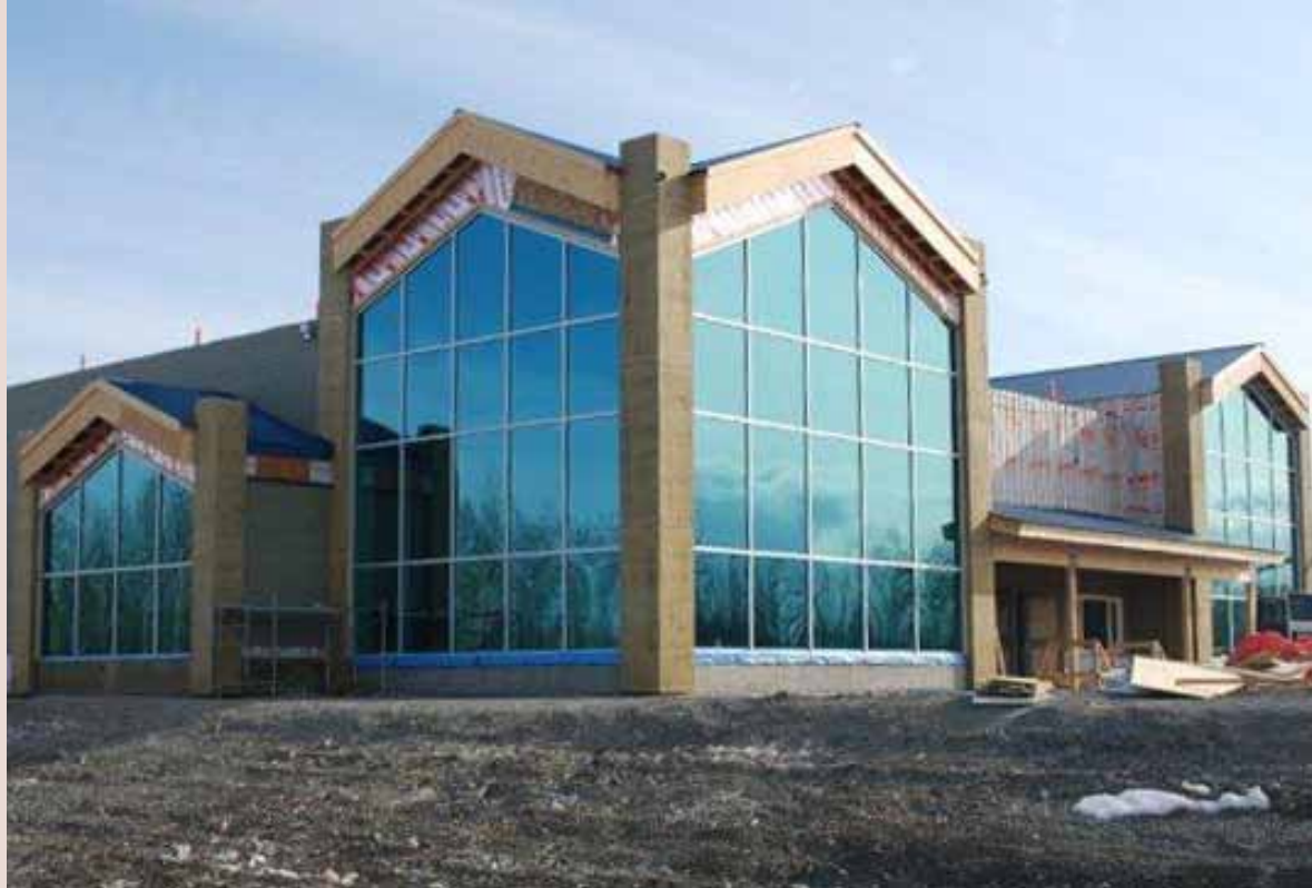
The first section of the Dä Kų Cultural Centre photographed this April. Construction of the main wing of the building will begin summer 2011.
